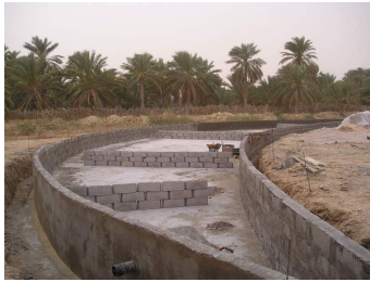
Figure 8b. Baffle walls to ensure sewage water’s proper residence time and avoid short-circuiting.
